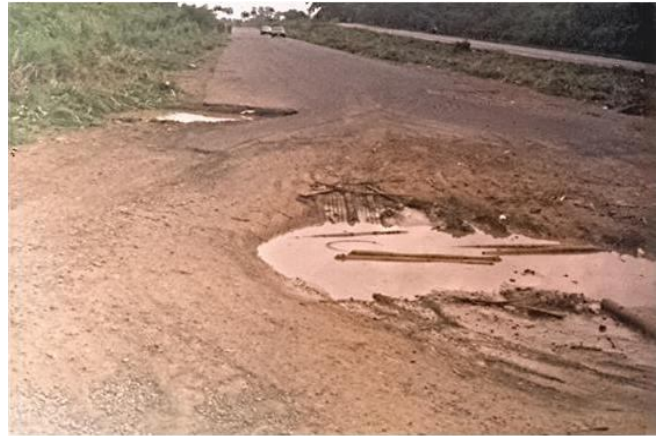
PLATE 2: Dangerous potholes, Lagos-Ibadan Expressway, Nigeria
