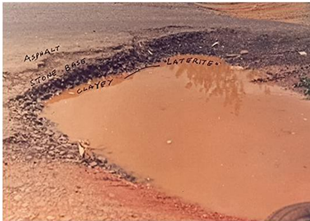
PLATE 1: Large pothole showing clayey lateritic, sub-grade, a stone base & the Asphalt wearing course on Lagos-Ibadan Expressway, Nigeria.
