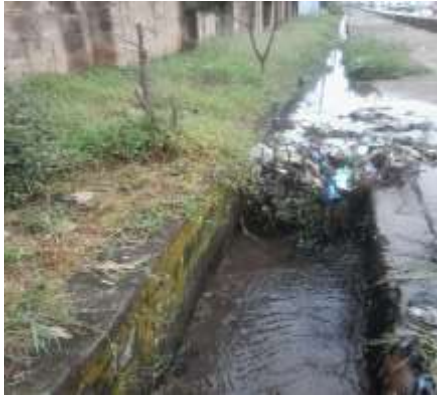
Figure 6: Waste disposed in drainages (Bauchi road)
