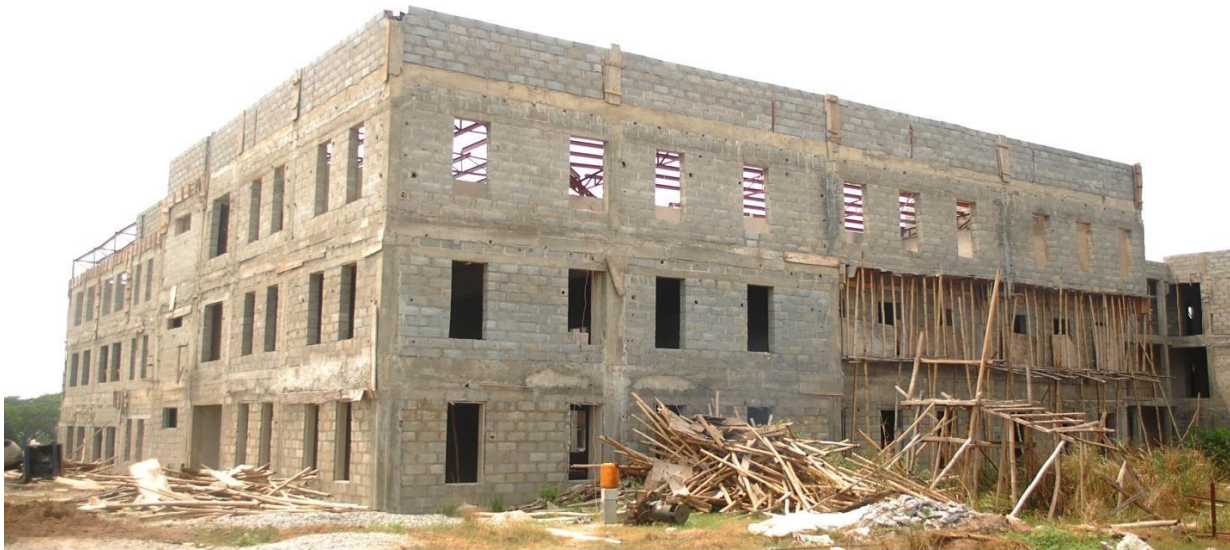
CONSTRUCTION OF ACADEMIC BUILDING COMPLEX (BLOCK A) - VIEWS OF RIGHTSIDE AND REAR
