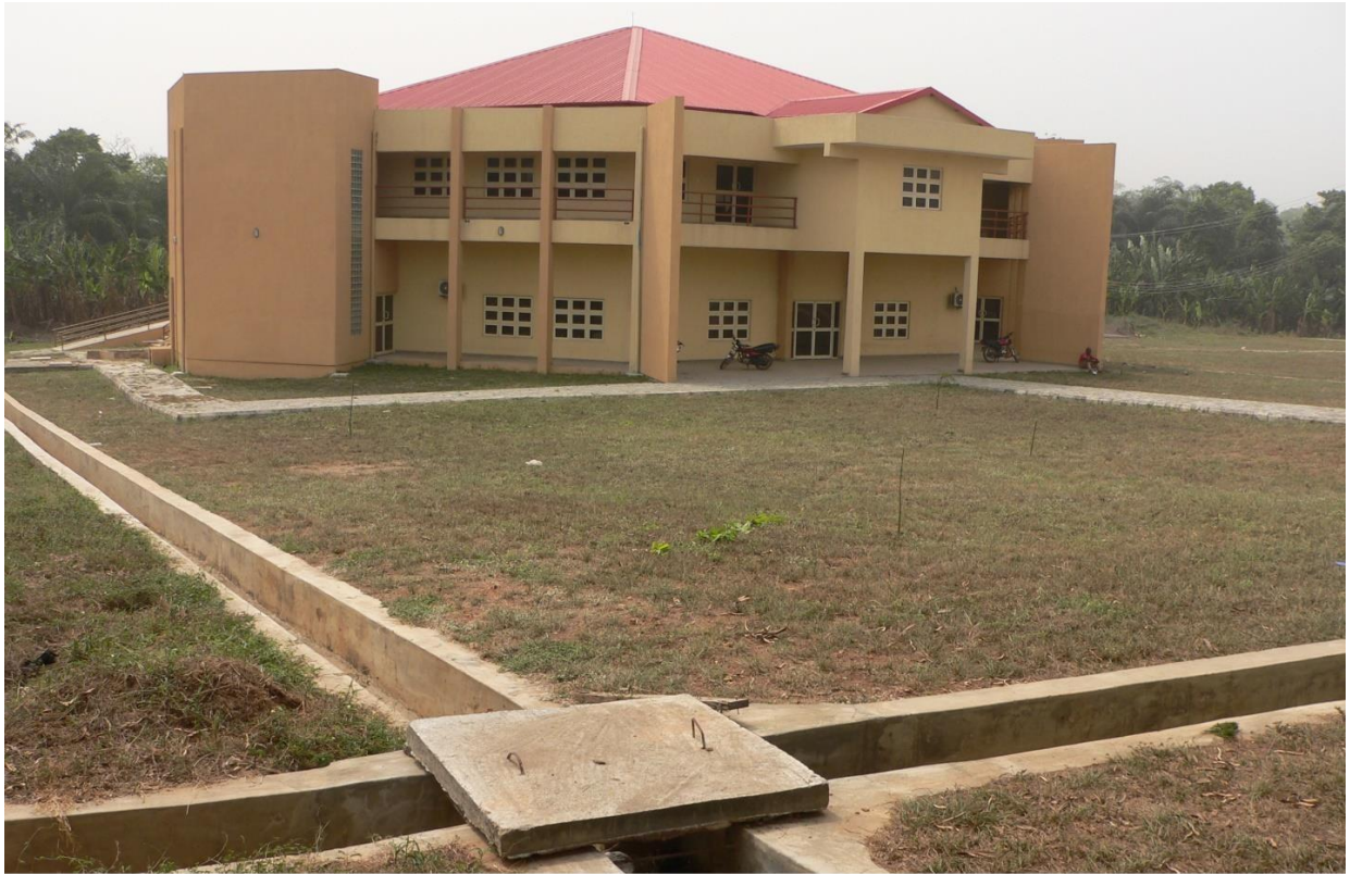
CONSTRUCTION OF CAR PARK, WALKWAYS AND DRAINAGE NETWORK FOR SCIENCE LABORATORY LECTURE THEATER
